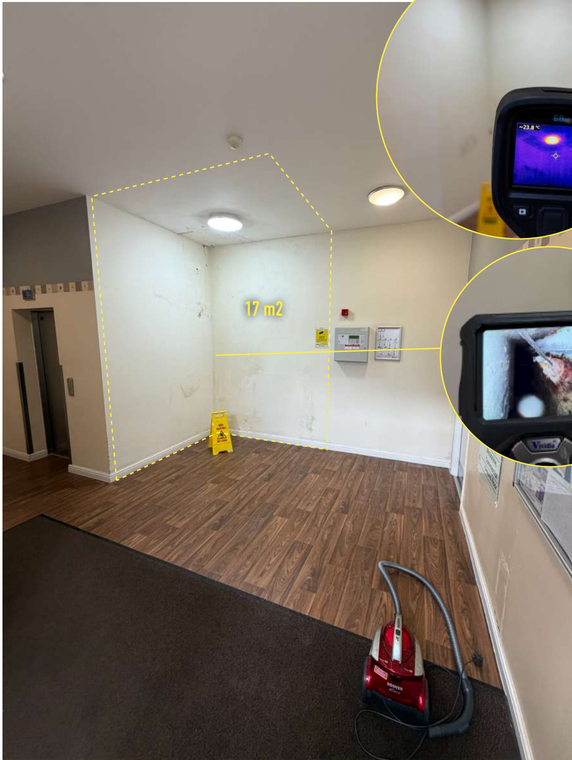
ENTRANCE LOBBY: The ceiling and walls show clear signs of water damage. Moisture testing confirmed that the affected areas are saturated, indicating ongoing water ingress rather than residual moisture from a historic leak. The lower image shows the rear face of the plasterboard with significant mould growth caused by prolonged moisture exposure. The plasterboard has been installed using the dot-and-dab method, resulting in isolated areas of higher moisture readings where the adhesive dabs are drawing moisture from the wall.
